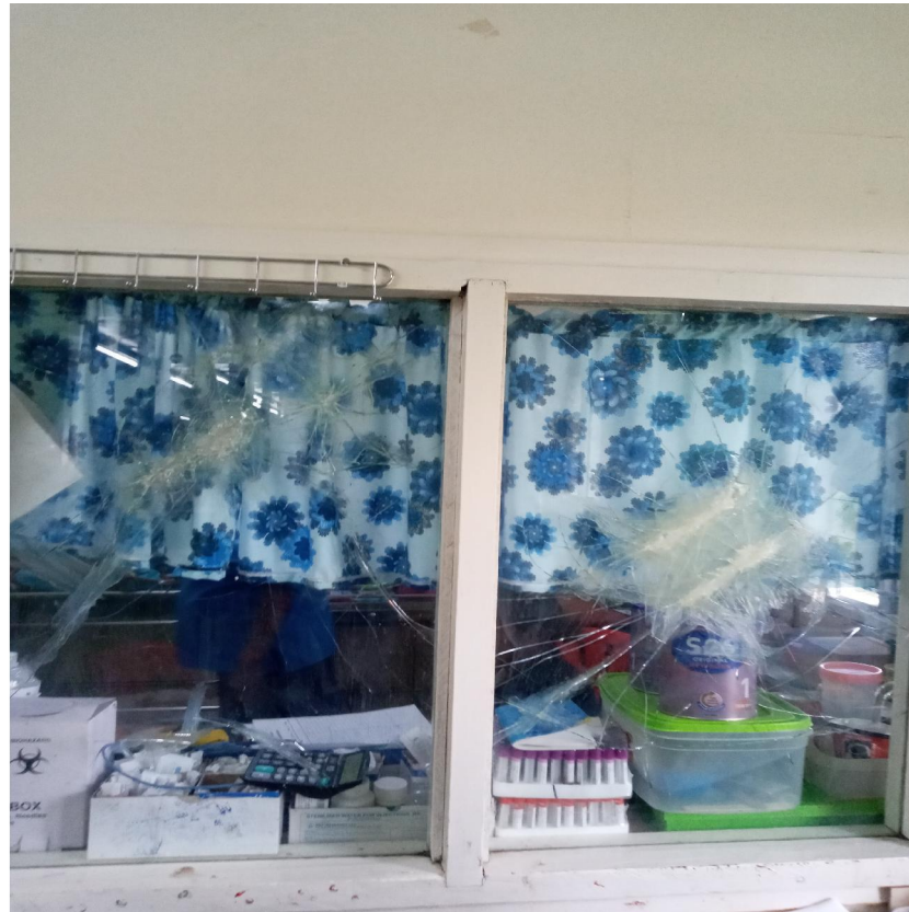
2017, post election rampage damages to SCN wall glass.
