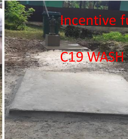
(f) Kaduwaga Pump final
